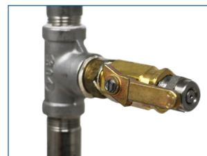
Two Zero-degree, 1/4in spray nozzles mounted on center tee fitting.
